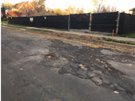
Westwood Street Pavement Failure, 10-30-23..jpeg 142K
